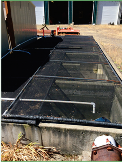
Chlorine Dosing System
