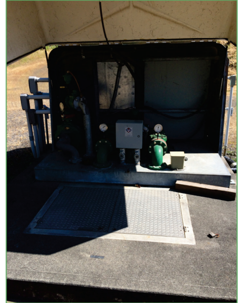
River Pump Station / Irrigation Pump Station
