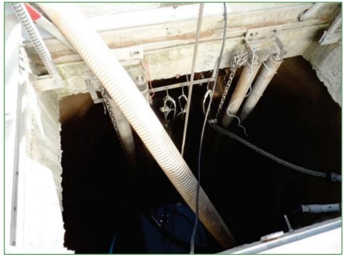
Return Pump Station
